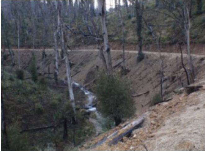
This is Rules Creek. The Yarrangobilly Caves water supply / hydro power pipeline is located underneath this track. The 1956 asbestos hydro line burnt or was damaged by falling trees in the fire. Some pipes needed to be retrieved from above the creek - a difficult asbestos clean-up task. As visitors drive down to the caves, they clearly view the replacement hydro line scar in the bush.
