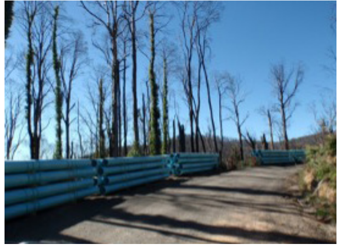
These are the replacement hydro line pipes. Due to the steepness of the site the pipes were stored on the Caves' Exit Road until the trench was dug. As the trench was located above the Entry Road this necessitated the closing of road for short periods so displaced rocks could not land on any vehicles.
