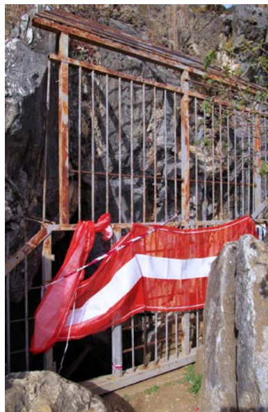
Figure 2 In 2017 and 2018 the entrance barrier was regularly damaged and at one stage, the gate was completely cut off and thrown into the cave.
