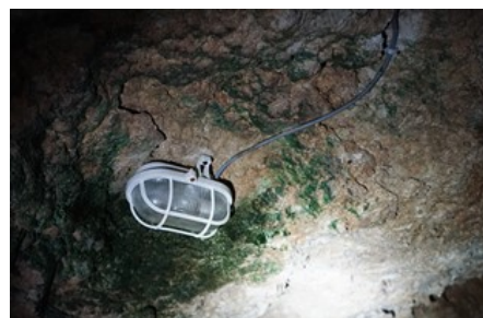
A simple bulkhead light fitting; functional but not aesthetic – with lampenflora
