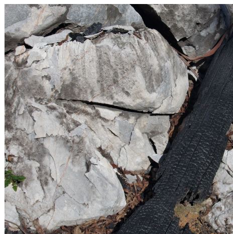
Figure 4 (below) Heavy spalling in close proximity to a burnt log.
